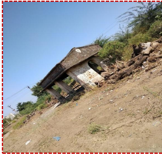
FIG.71 THORDI OLD SMASHAN WHICH SHOULD BE CONSTRUCTED NEW
